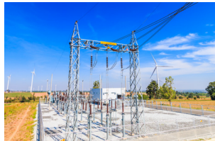
Substation partial discharge
